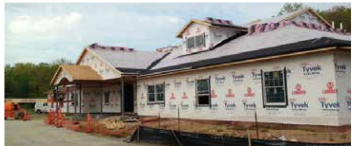
Roofing material, including shingles donated by Owens Corning, were scheduled to be added beginning the week of May 15 th .
