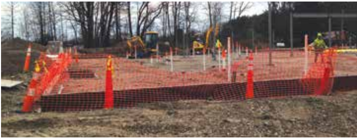
In early April the foundation was completed and the underground utilities installed. An insulation layer and vapor barrier were installed before pouring the concrete floor.
